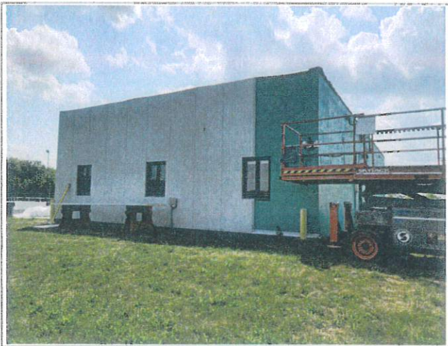
Closer view of east face of the building showing progress of panel installation. Panels weigh approximately 250 lbs each.
