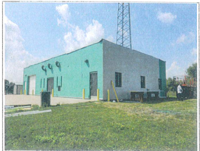
Overview from SE corner of site, shows crews progressing with IMWP installation along the east face.
