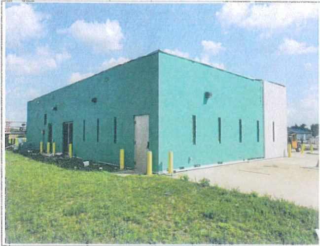
Overview from NW corner of site, shows a couple of panels have been installed on the west face of the building.
