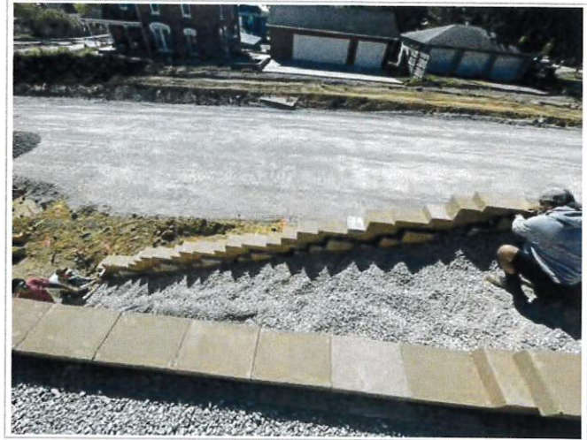
Kevin's Concrete pulling string line for the stairs located in the retaining wall
