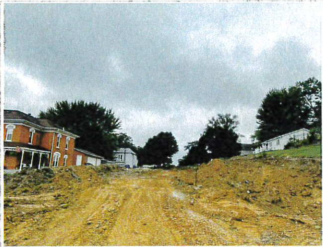
PCI has street removed west of Greene and working towards Washburn Street
