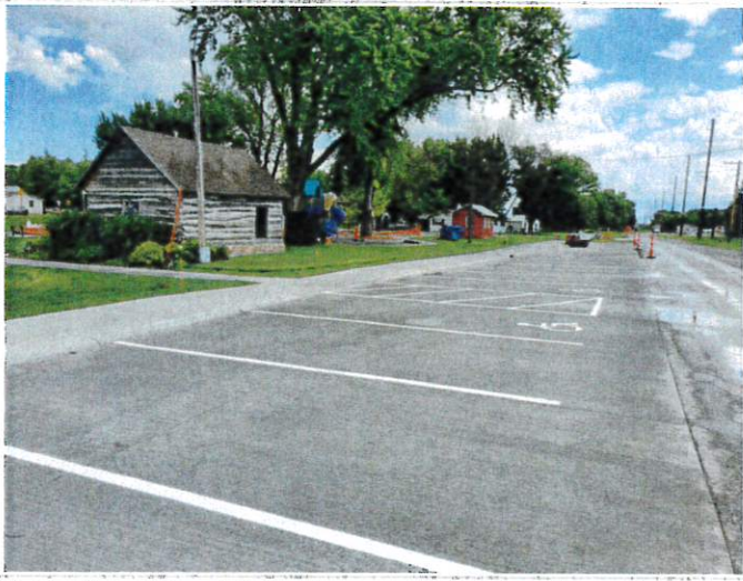
Striping for parking stalls has been completed along the east and south parking areas, Handicap signs still need installed
