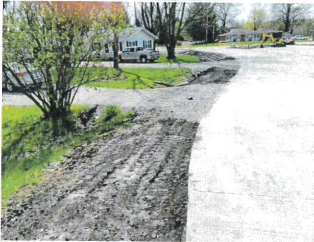
The (2) driveways along S Hickory have been graded to street level and road/ditches have been backfilled
