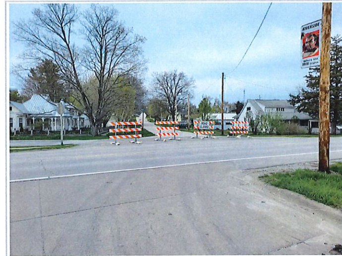
Road closure signs have been set throughout the project, view of Rose and HWY 22
