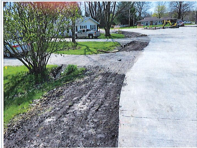
The (2) driveways along S Hickory have been graded to street level and road/ditches have been backfilled
