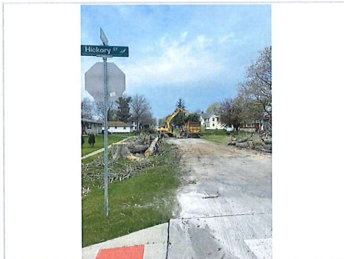
Looking west down Third Street shows trees are down and debris being removed
