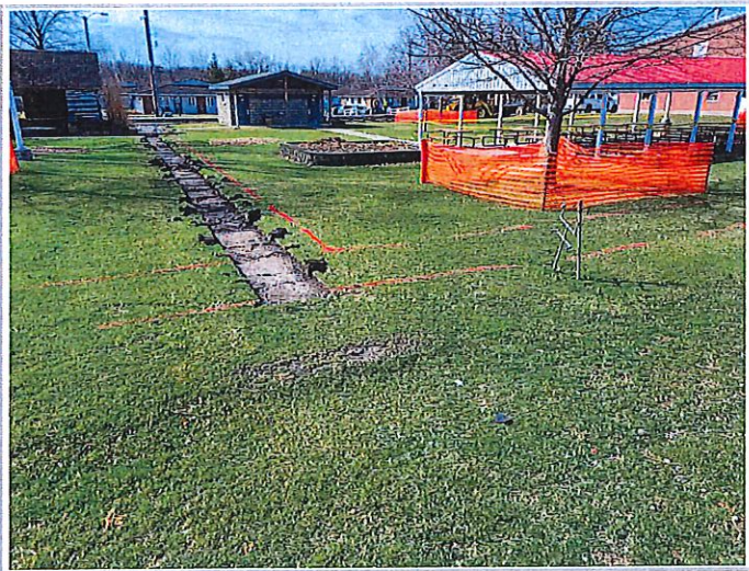
New sidewalk has been marked out throughout the park - view of work completed in center of park
