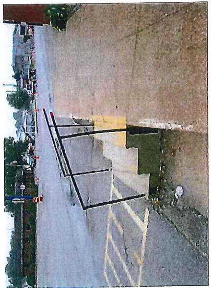
SIDEWALK SAFETY The drop-off of the downtown sidewalk on the north side of Highway 22 poses a significant safety threat and should be addressed immediately.
