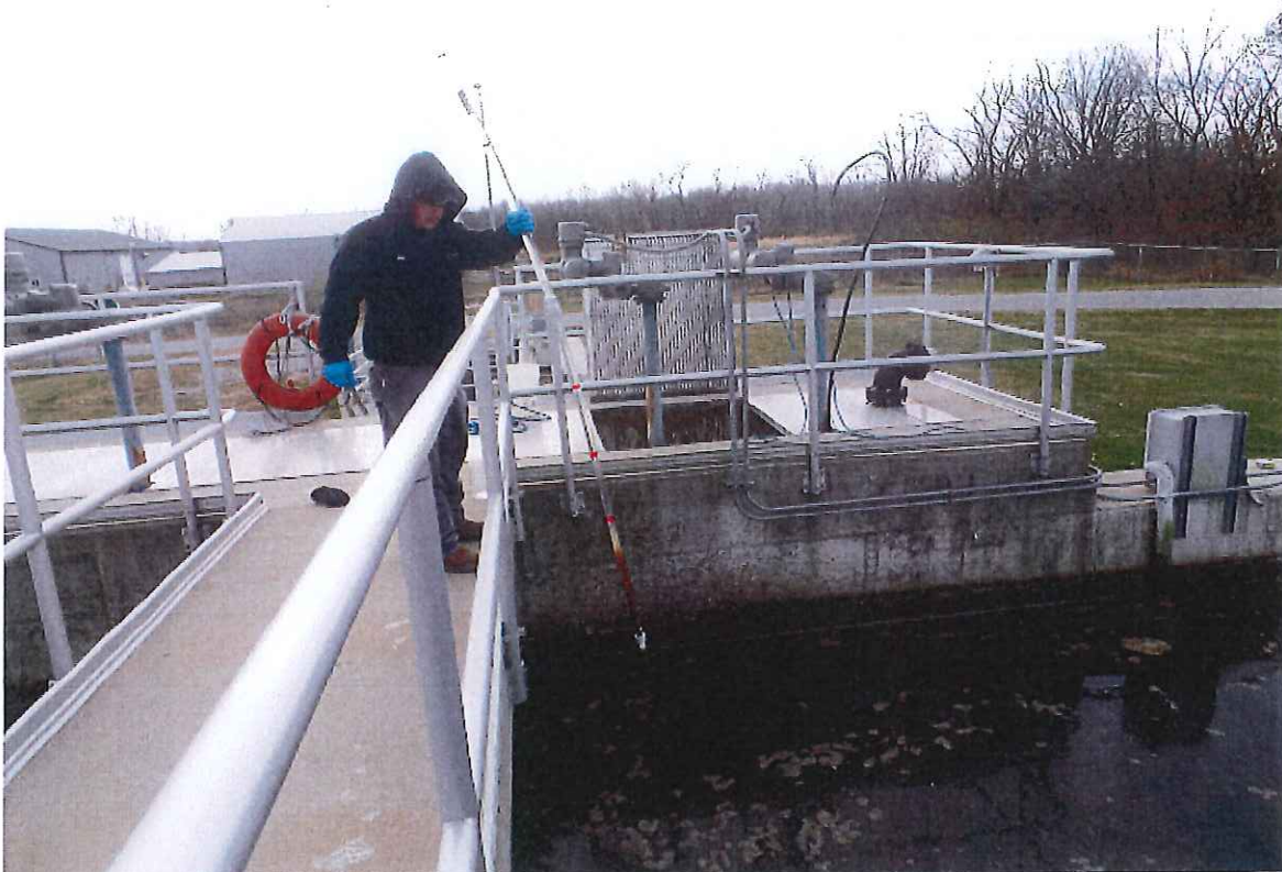
SBR 1 Sludge Core – Blanket Level 9.5 ft., Very Clear Supernatant
